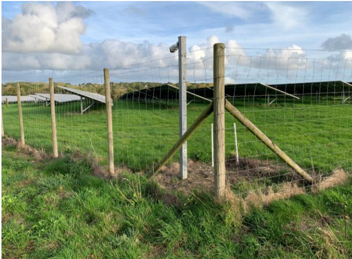
Photos 42 and 43: CCTV Poles and Fencing
